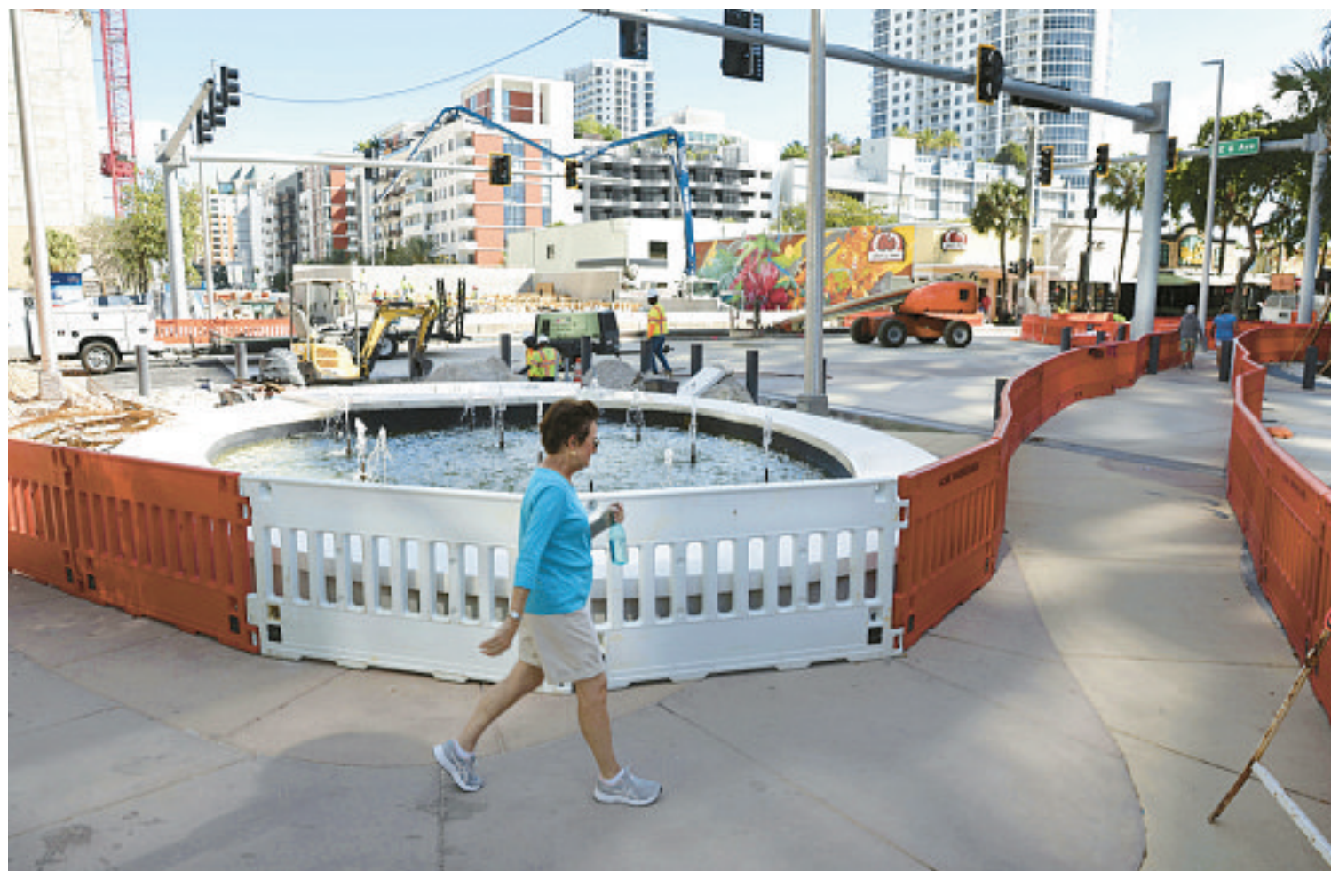
A woman walks Thursday by the park being built along Las Olas Boulevard on top of the Henry E. Kinney Tunnel in downtown Fort Lauderdale. Work on the park is expected to be finished in late May. CARLINE JEAN/SOUTH FLORIDA SUN SENTINEL
