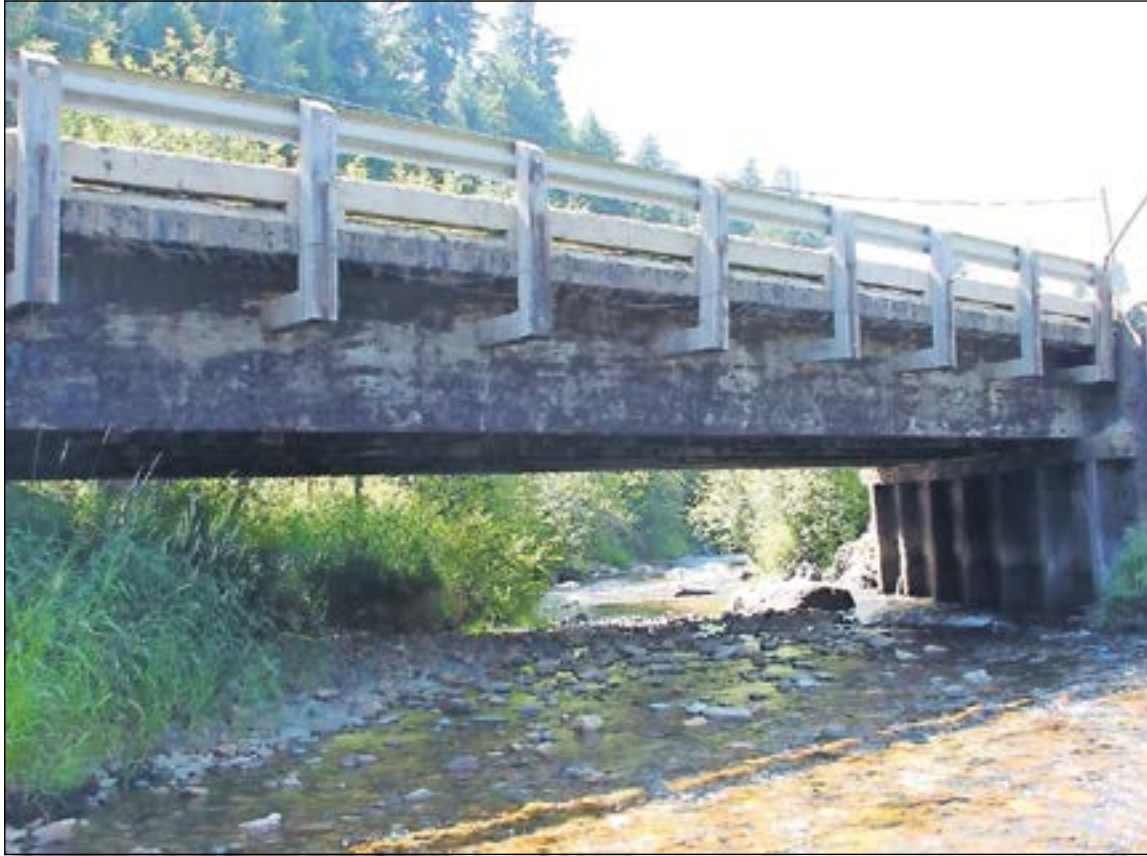
Bonner County Road & Bridge officials are seeking public comments on a project to replace an aging span across Rapid Lightning Creek.
